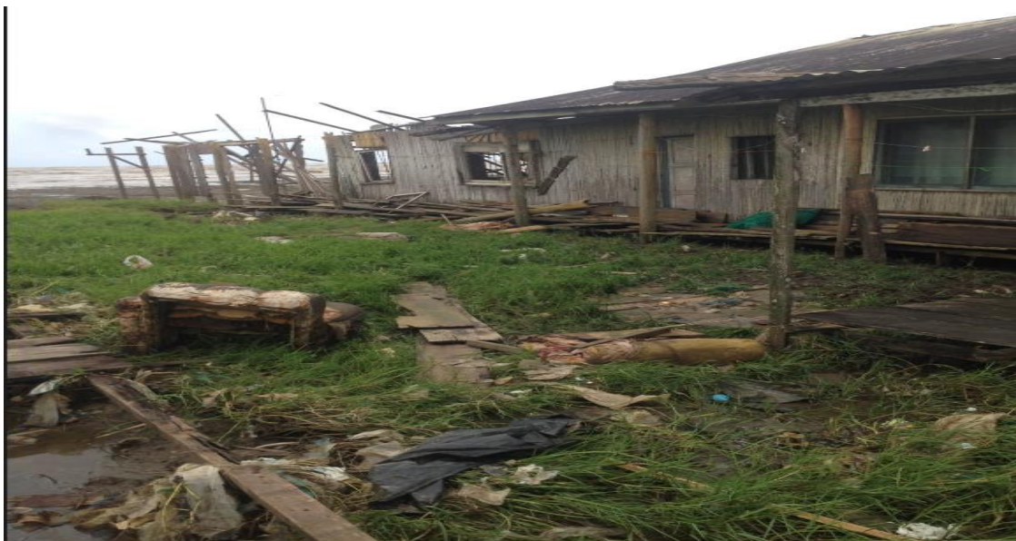
Figure 6: Destruction of building Infrastructure in Ayetoro
