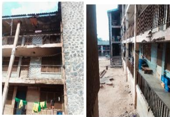
Plate 4: Crack walls and room condition from the front view
